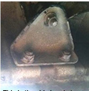
This is the side bracket (one each side) these need to be removed and our relocation plates inserted, for the 3" and 4" lift this bracket has to be flipped (turned upside-down) Note that the spacers DO NOT sit on the chassis mount point!
